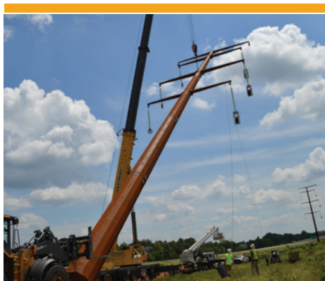
Crews set a structure near Holmen, Wis., on the CapX2020 345-kV transmission line. Courtesy of CapX2020.
